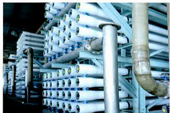
Reverse Osmosis System
