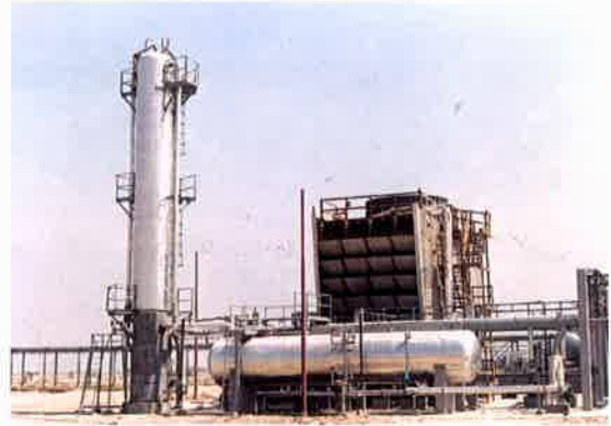
Effluent Treatment Plant for IFFCO-Aonla
