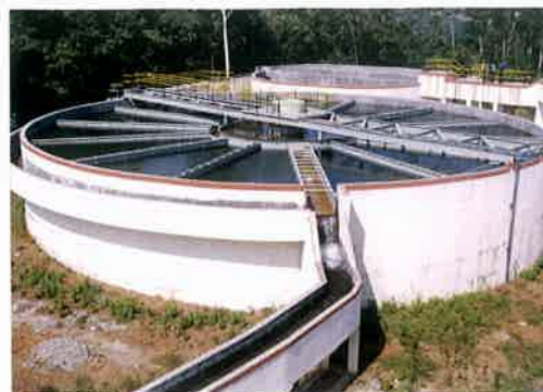
40 MLD WTP, Curti-Ponda , PWD, Goa
