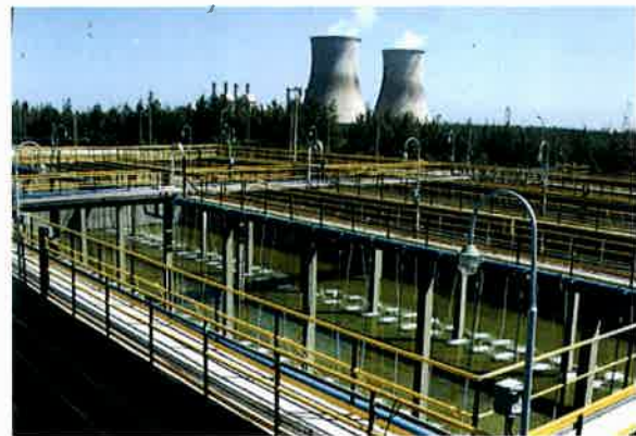
Diffused Aeration based Effluent Treatment Plant including Tertiary Treatment for reuse of waste water for Reliance, Hazira
