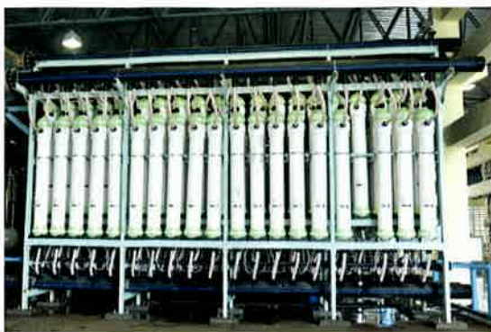
Ultra Filtration System
